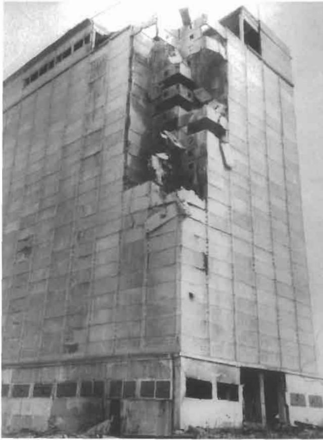
Figure 2.20 Corner of the silo complex in Tomylovo, USSR, damaged by smoldering gas explosions, 1987–1989 (Courtesy of A. Borisov and B. Gelland, USSR Academy of Science, Moscow).
