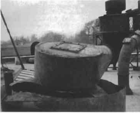
Figure 1.99 Damaged cyclone after a dust explosion. The vent cover was too strong to open before the cyclone itself ruptured (From Department of Employment and Productivity, 1970).
