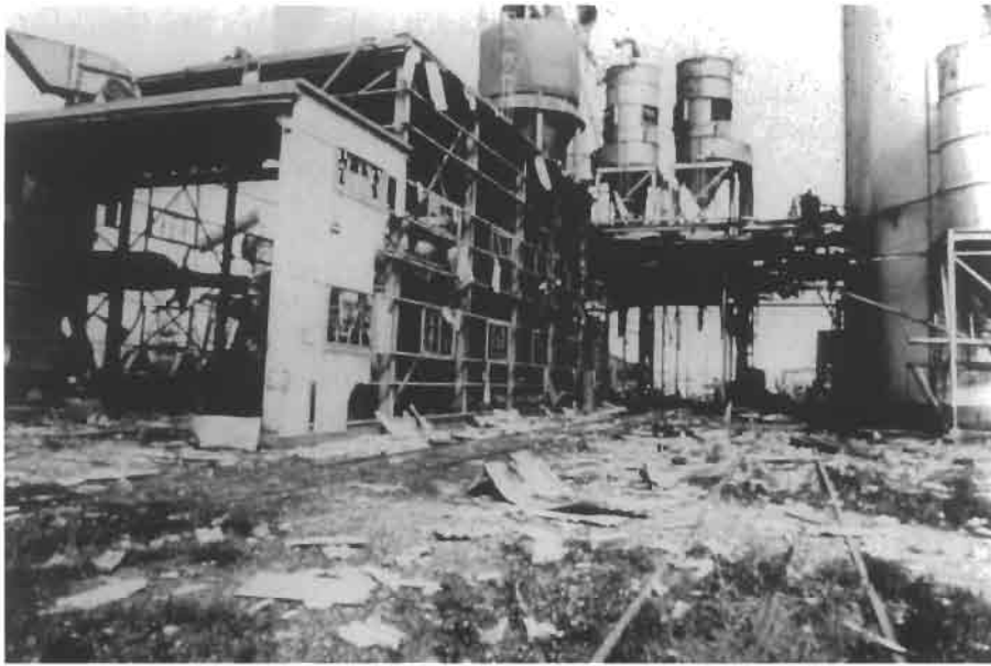
Figure 2.14 Destroyed dump area of the Corpus Christi grain silo plant after major grain dust explosion in 1981 (Courtesy of C. W. Kauffman, University of Michigan).
