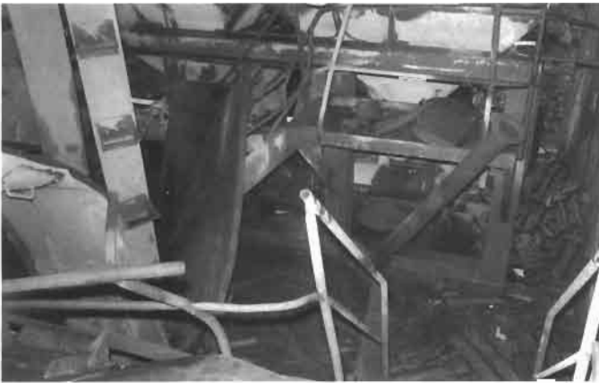
Figure 2.28 Detailed view of the extensive material damage cause by the silicon dust explosion at Bremanger, Norway, October 1972.
