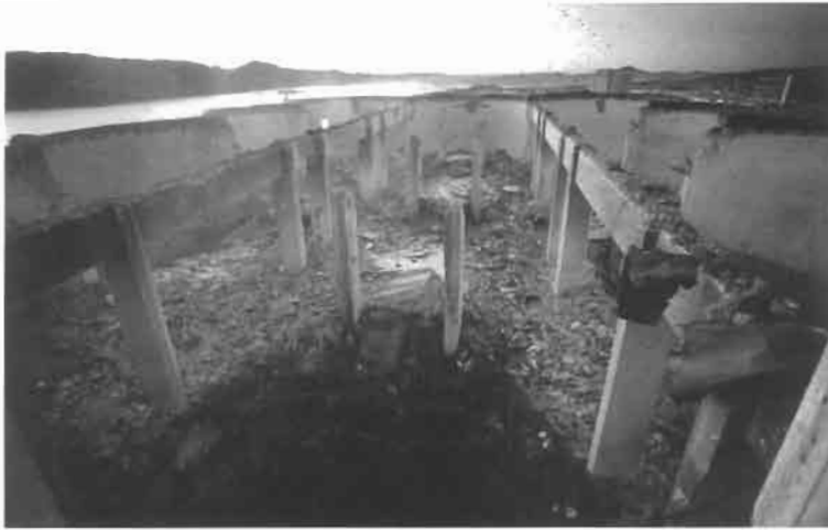
Figure 2.19 View of damaged loft of silo plant in Stavanger, Norway, after smoldering gas explosion in November 1985 (Courtesy of Øyvind Ellingsen, Stavanger Aftenblad, Norway).
