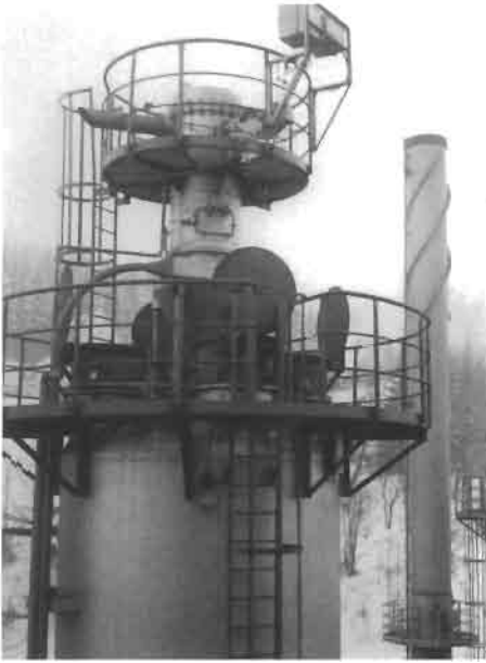
Figure 1.105 Reversible, low-mass hinged explosion doors (see Figure 1.104) installed in the roof of a silo (Courtesy of T. Pinkwasser, Bühler, Switzerland).
