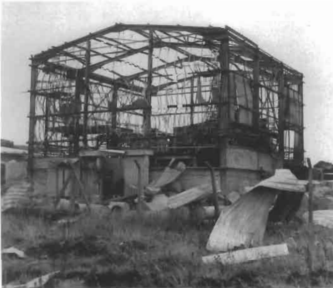
Figure 2.35 Damaged screen room after a dust explosion in an aluminum powder production plant at Anglesley, United Kingdom, in 1983 (Courtesy of G. Lunn, Health and Safety Executive, United Kingdom).
