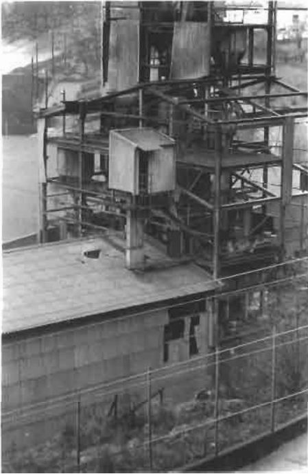
Figure 2.27 Totally destroyed milling section of silicon powder production plant at Bremanger, Norway, after the dust explosion in October 1972.
