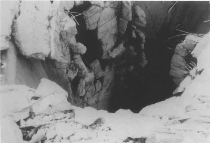
Figure 2.9 Air shaft along the damaged walls of reinforced concrete silo cells of the grain terminal at St. Joseph, Missouri, 1980 (Courtesy of C. W. Kauffman, University of Michigan).
