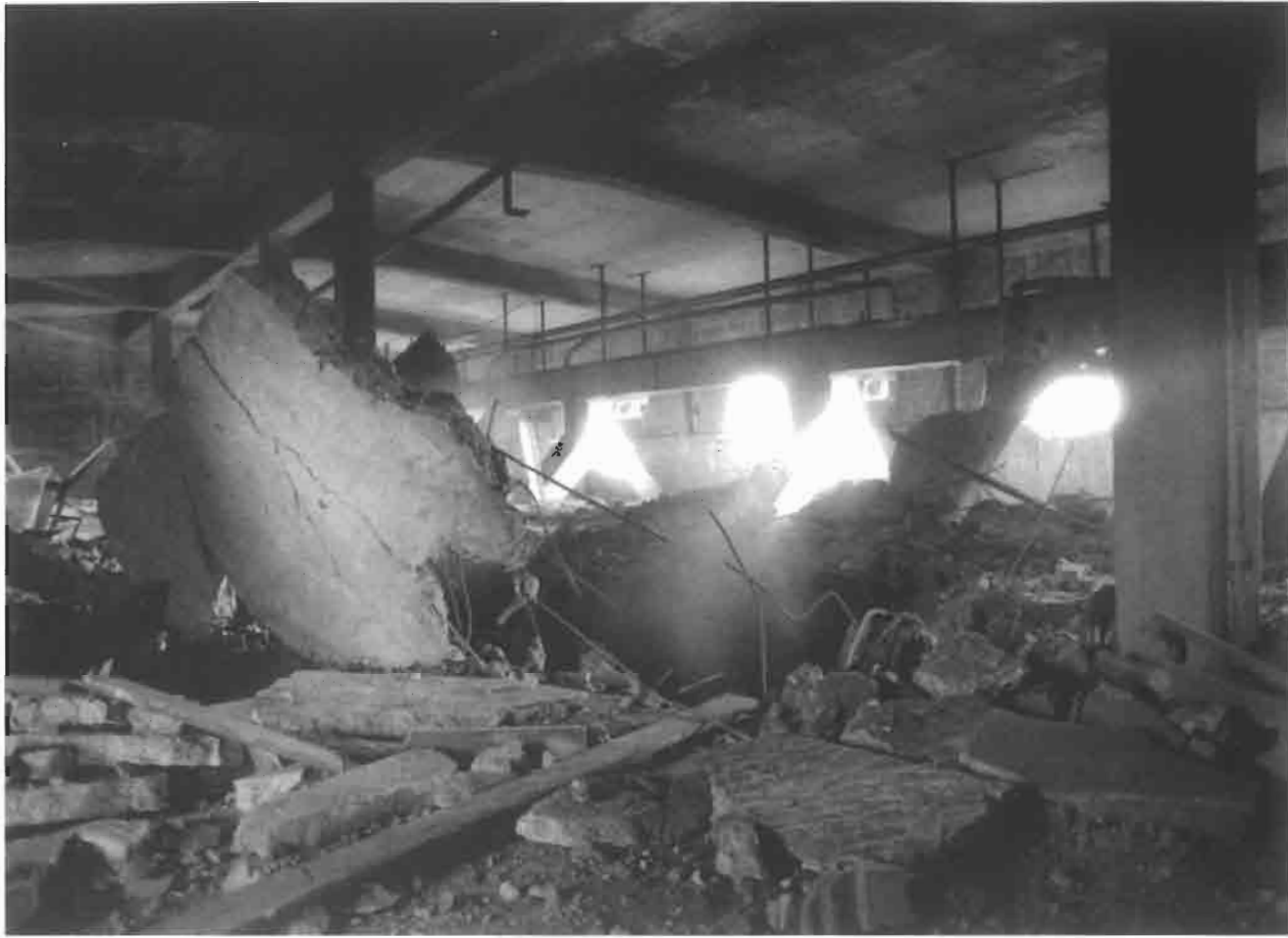
Figure 2.23 Damaged silo roof after a smoldering gas explosion resulting from smoldering wheat bran pellets in a 39 m tall concrete silo in Malmö in 1989 (Courtesy of C. Templin and B. Persson, Nord Mills, Sweden).
