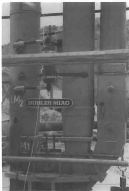
Figure 1.126 Application of automatic dust explosion suppression to bucket elevators (Courtesy of T. Pinkwasser, Bühler, Switzerland). For a much clearer picture, see Color Plate 4.
