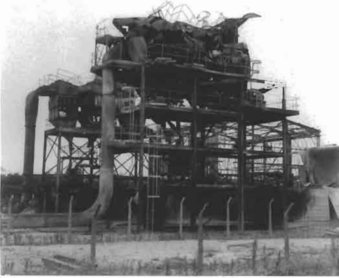
Figure 2.34 Damaged no. 2 stream collectors after a dust explosion in an aluminum powder production plant at Anglesley, United Kingdom, in 1983 (Courtesy of G. Lunn, Health and Safety Executive, United Kingdom).
