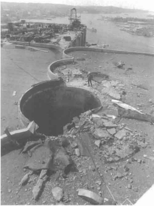
Figure 2.2 Damaged silo roof after the wheat grain dust explosion in Stavanger in June 1970 (Courtesy of Egil Eriksson).
