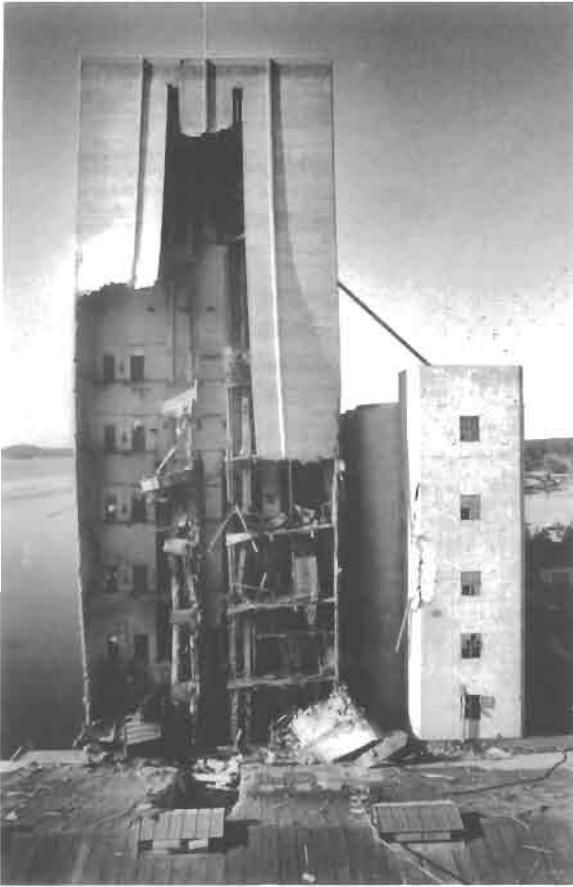
Figure 2.6 Damaged silo head house after a grain dust explosion at Kambo, Norway, in June 1976 (Courtesy of Scan Foto, Oslo, Norway).
