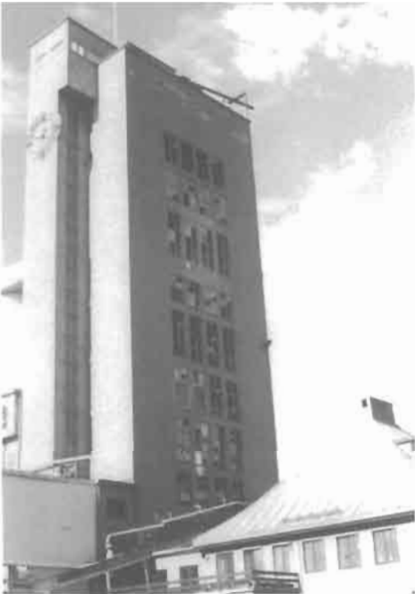
Figure 1.135 Result of malted barley dust explosion in grain silo facility in Oslo, Norway, in 1987. The windows provided sufficient venting to prevent destruction of building, which is of reinforced concrete (Courtesy of A. F. Johansen, Oslo Port Silo, Norway).
